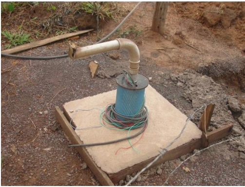
Figure 3 - Well with flow 7 m 3 / h , for community supply
